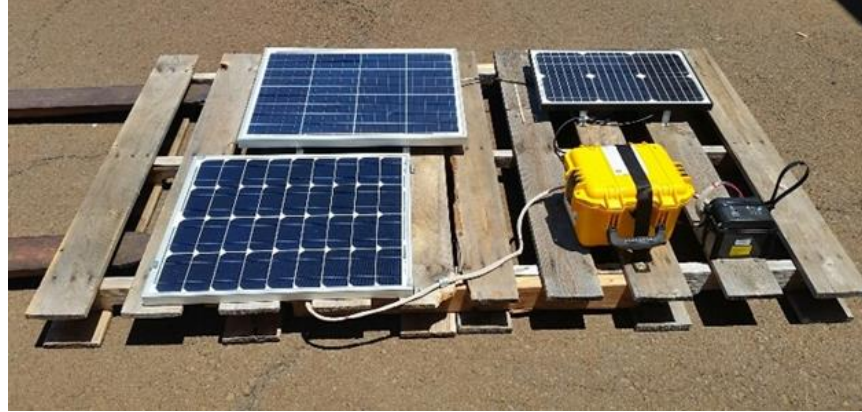
Figure 2. The assembled test system in the field. The polycrystalline solar panel is positioned at the top right with the monocrystalline panel below it. The yellow waterproof case is present as well. The external battery and the third panel to charge the battery are each in the bottom right and top right of the photo, respectively. [4], [9]
